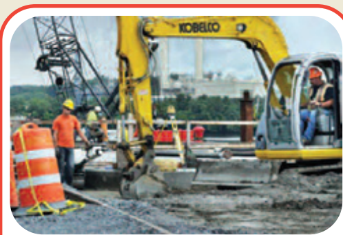
Workers finish new railroad tracks on the south end of the new wharf new Shed 5 at the Port of Albany Tuesday Aug. 16, 2011. Work is winding down and should be completed in September. (John Carl D'Annibale / Times Union)
